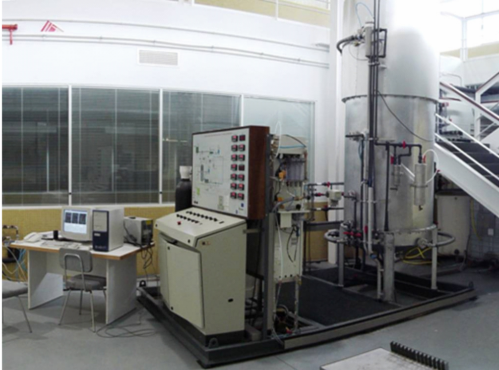
Figure 4.8. Anaerobic pilot plant placed in the School of Engineering at the University of Santiago de Compostela. Hybrid UASB-AF reactor, pumps, piping, sensors, control panel, monitoring and data acquisition system.
