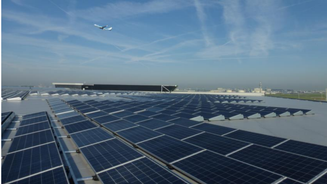
FIGURE 4 PARK 20|20 SOLAR PARK
