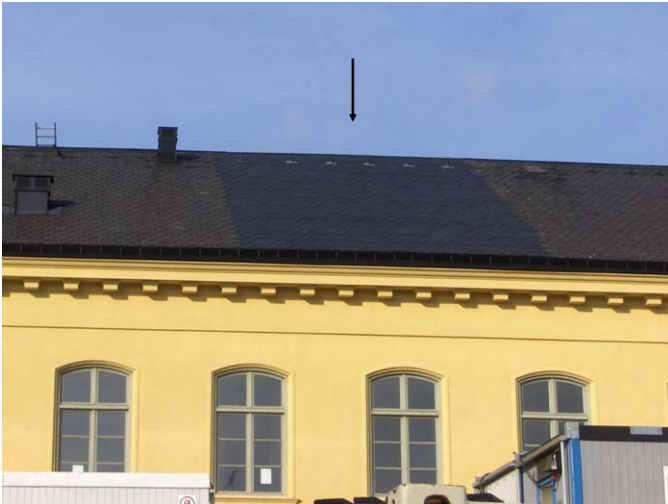
Fig. 1. Example of inadequate partial replacement of roofing slate.
