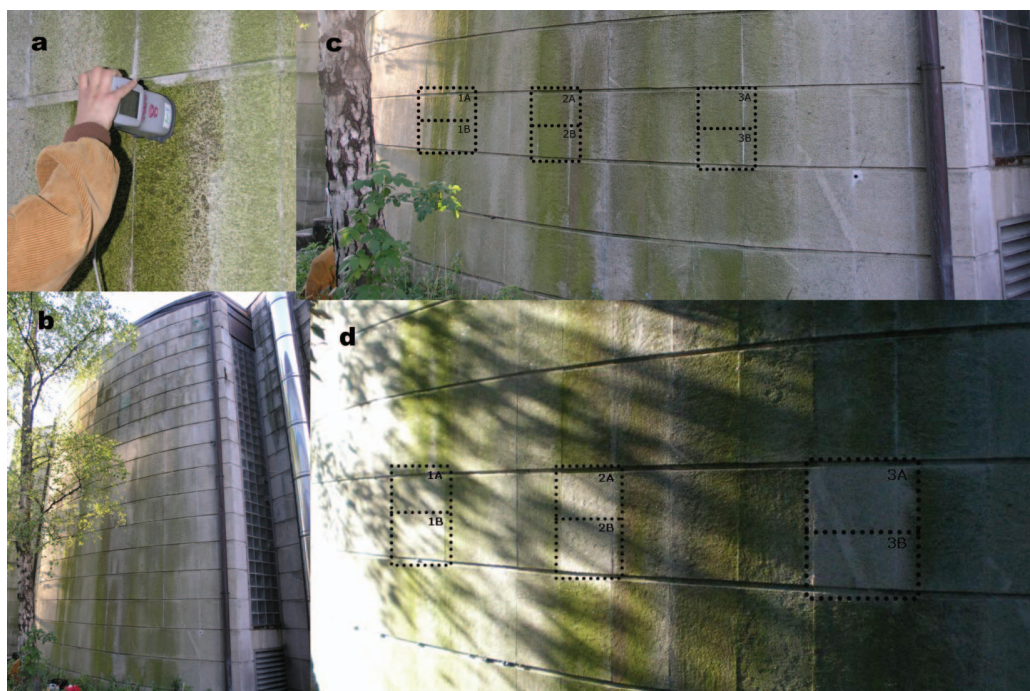
Figure 1. Granite façade of the Supercomputing Centre of Galicia (CESGA), showing extensive phototrophic colonization (greening) developed as streaks following the path of water run-off. (a) On site measurement of the color on the façade; (b) overview of the façade with perceptible colored stains (greening) in humid zones; (c) location of the six study areas before cleaning; (d) location of the six study areas after cleaning. Six study areas: three target areas (1, 2, 3) each of which was divided in two subareas, upper (A) and lower (B).
