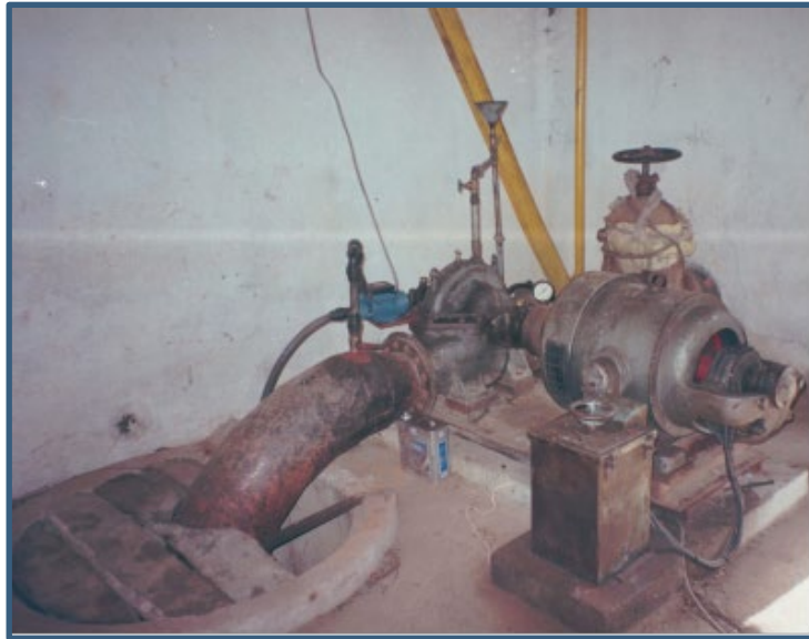
Image 4.2.2.12. Obsolete water pumping equipment, River Lea
