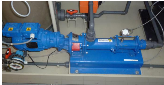
Figure 9. Recirculation pump (P-1102)
