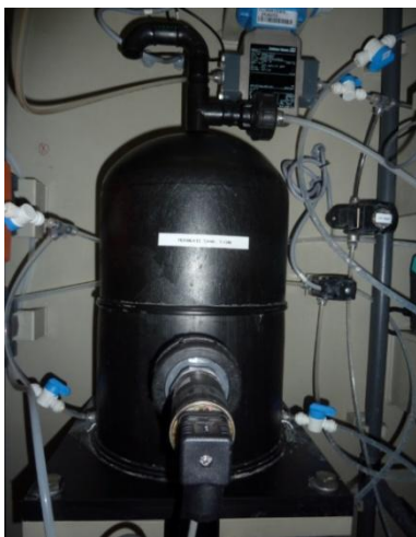
Figure 33. Old permeate tank (T-1700)
