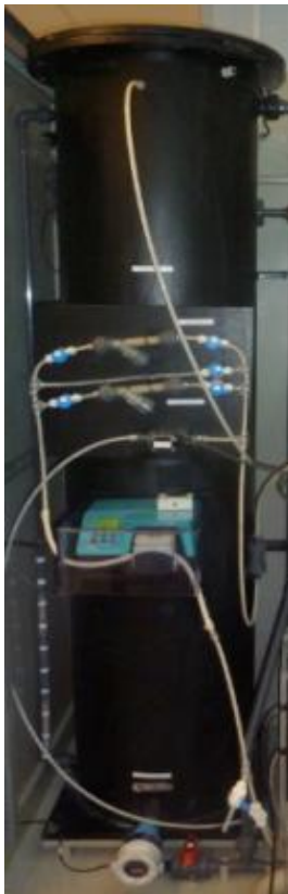
Figure 15. Buffer Tank (T-400)
