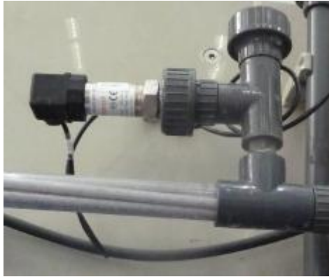
Figure 20. Permeate pressure sensor (PT-1604)
