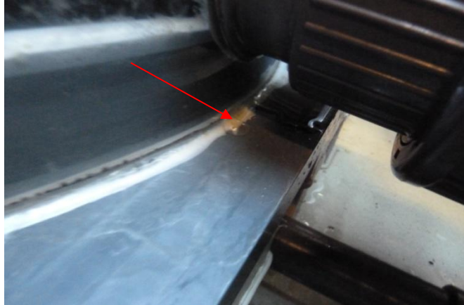
Figure 27. Water leaking detected at the bottom part of the jacket reactor
