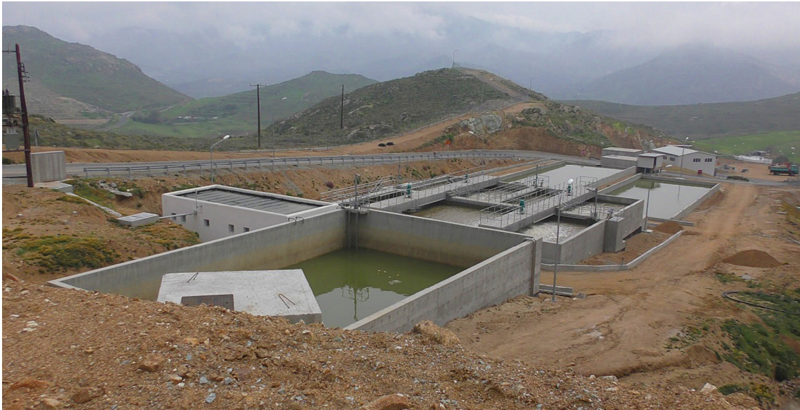
Figure 61. Waste water treatment plant in Naxos.
