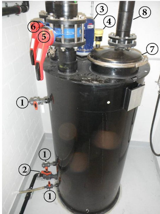
Figure 5.2. Urine storage tank, at the basement of EAWAG office building. 1) Sample ports. 2) Effluent port. 3) Mixer. 4) Level sensor. 5) Women's toilet influent. 6) Men's toilet influent. 7) Hermetic tight. 8) Ventilation.
