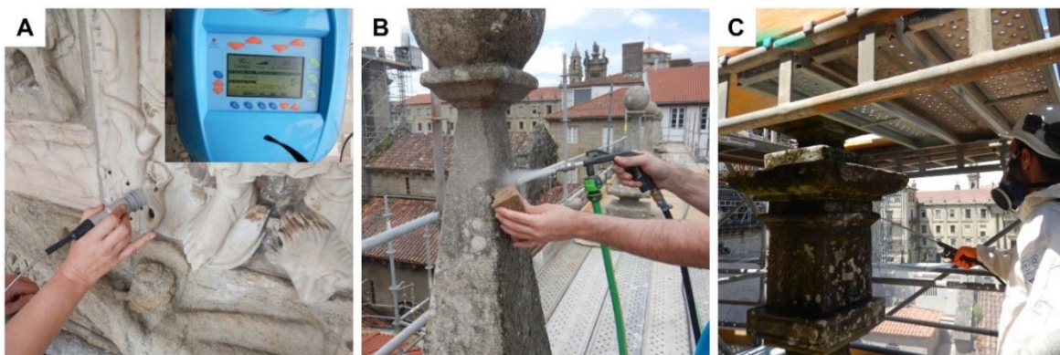
Figure 35. Photographs showing examples of the three cleaning methods evaluated in the current study. a) Application of laser cleaning, with inset showing detail of the device (image provided by Parteluz Estudio S.L.). b) steam application (image provided by Parteluz Estudio S.L.). c) application of chemical biocides (image provided by María Gómez García, restorer).
