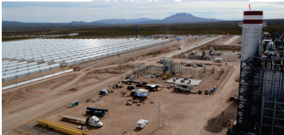
Fig. 9 Agua Prieta II Hybrid Power Plant. [18]
