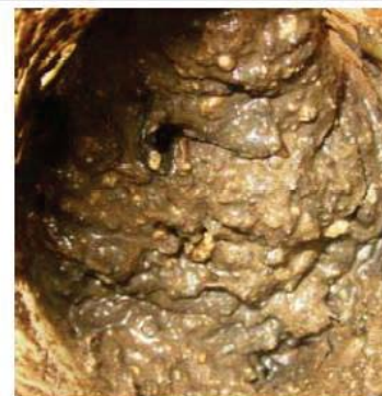
Grasa DAF EDAR Guillarei
