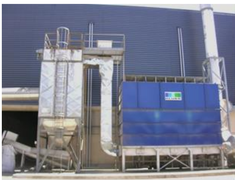
Figure 5.2. Bag filter and regenerative thermal oxidiser
