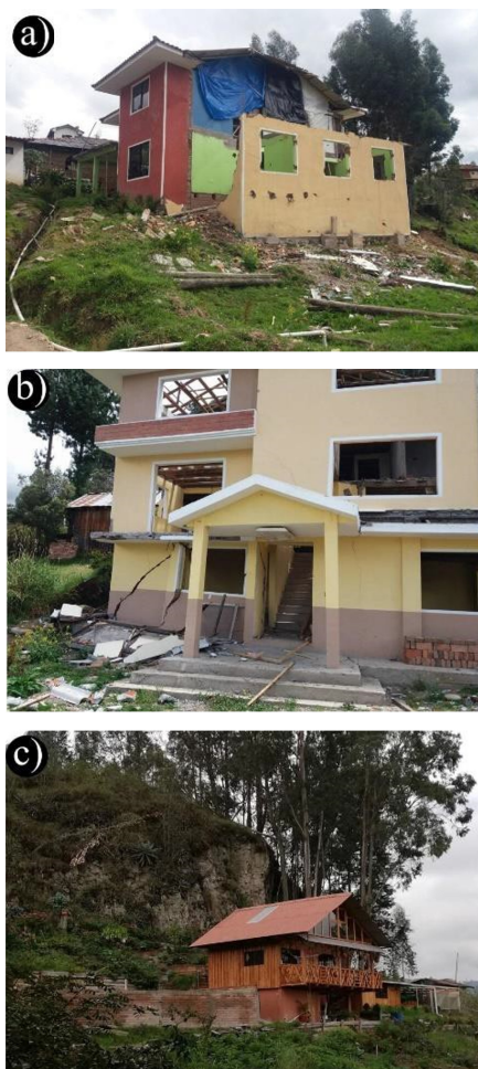
Figure 2.2: a) House completely destroyed by a mass movement; b) house with considerable disjunction, floors inclined and walls out of plumb due to a landslide; c) an example of low-risk perception by the local population. The structure was built close to a subvertical rock wall which is very prone to mass movements such as rockfalls, topples and slides (photo: M. Ramondini).
