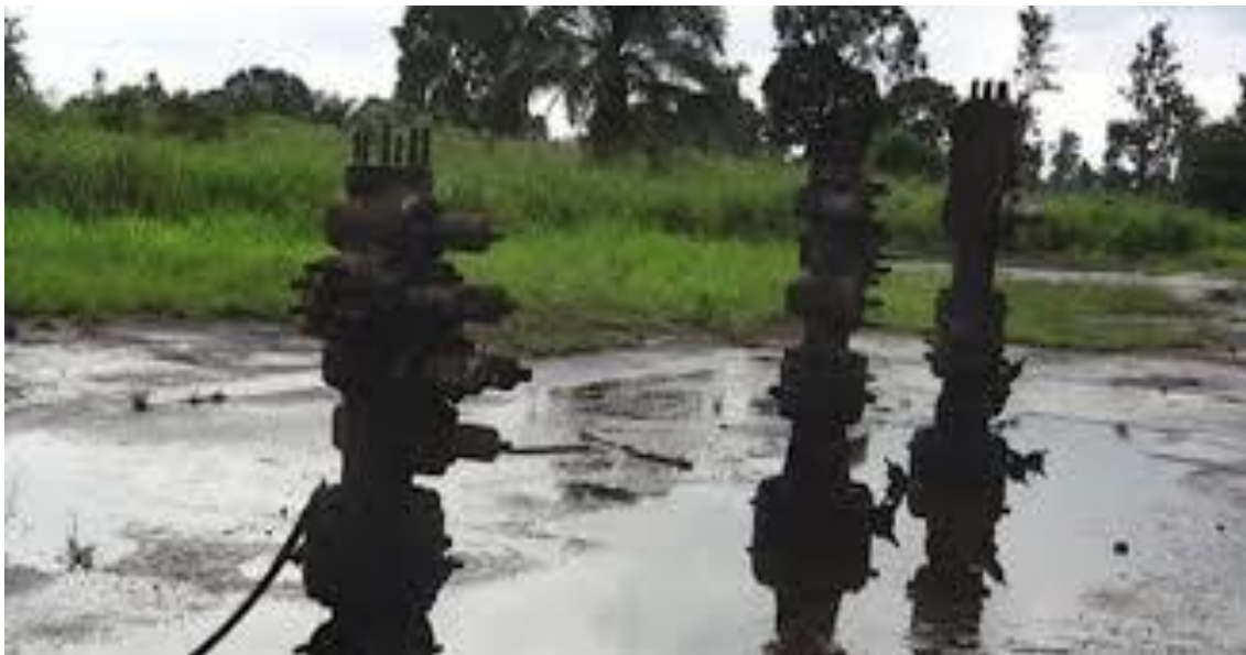
Figure 20: Oil Leakage at Eleme Refining Well – Rivers State.
